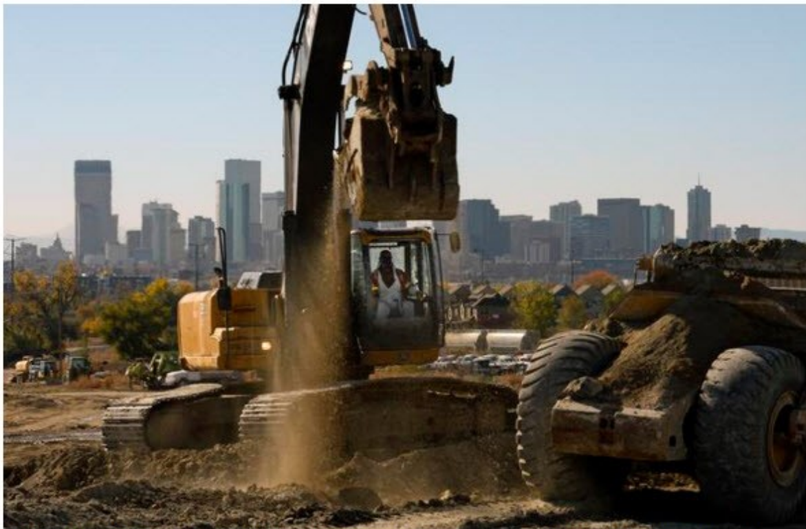
Work continues Wednesday at the 77-acre site of the former Asarco smelting plant in Denver. (Helen H. Richardson, The Denver Post )
